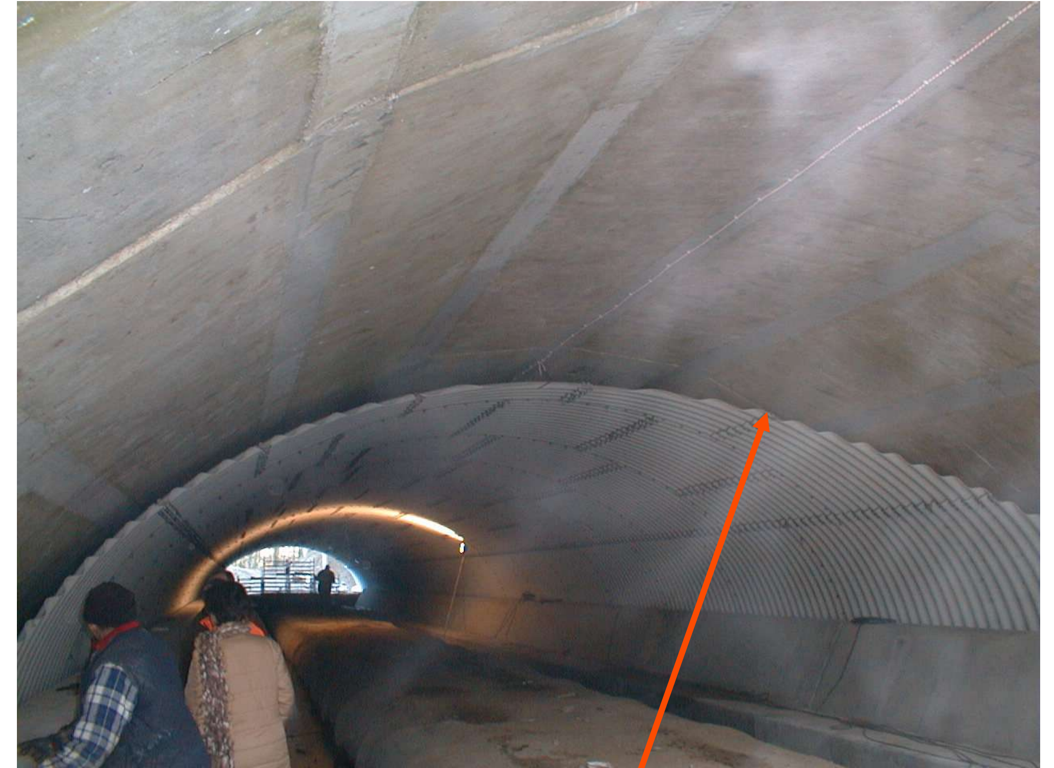
dimensioning of new structure as close as much to the existing cross-section
